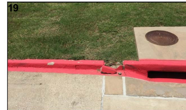
Broken Curb & Gutter - Replace Curb & Gutter
