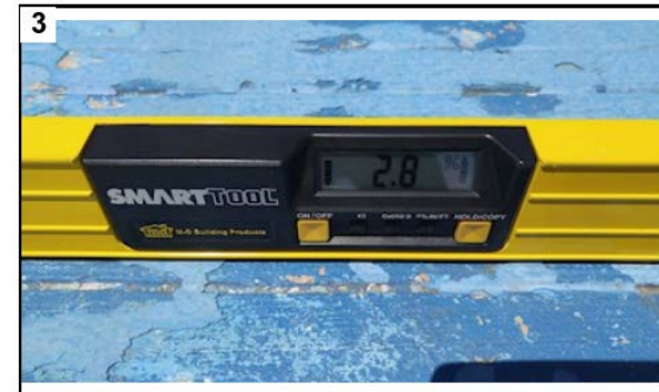
Running slope of curb ramp is 9.3%, which exceeds maximum allowable slope of 8.3%.
