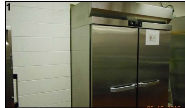
The pass-thru heated cabinet has broken knobs and the temperature cannot be controlled. Unit is very old.
