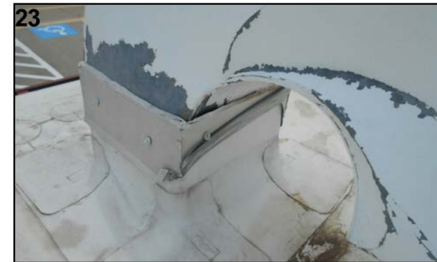
Counterflashing metal bent up and unsealed.
