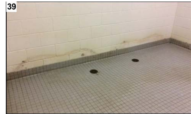
Water stains at lower section of wall.
