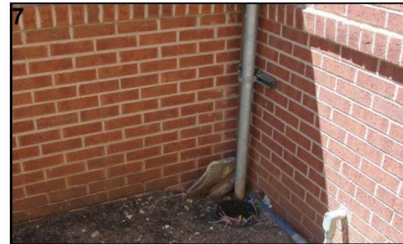
Loose cabling to be covered, removed or installed in a conduit pathway and terminated at its proper location. All abandoned cabling must be completely removed per the National Electric Code.
