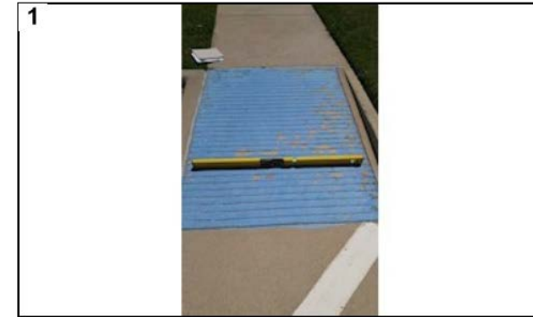
Curb ramp cross slope of 2.3%. Maximum allowable 2%. Slope of 2.3% is within generally accepted tolerance for existing facility.
