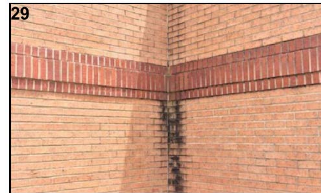
Roof edge drainage is causing water stains to wall below.
