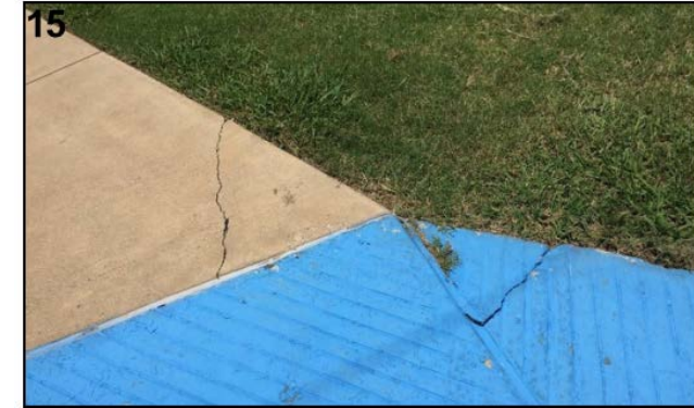
Broken Pavement - Replace Pavement
