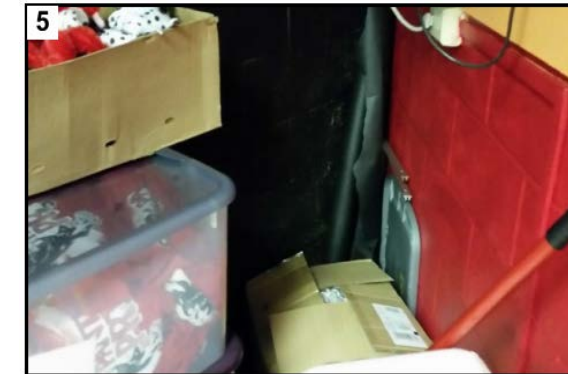
b. The space is shared leaving the IDF inaccessible due to stored items.
