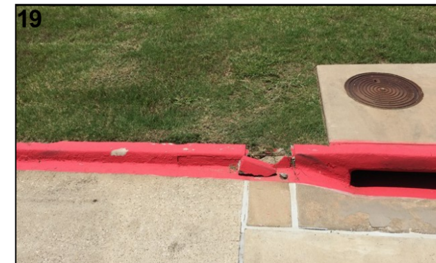
Broken Curb & Gutter - Replace Curb & Gutter
