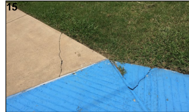
Broken Pavement - Replace Pavement
